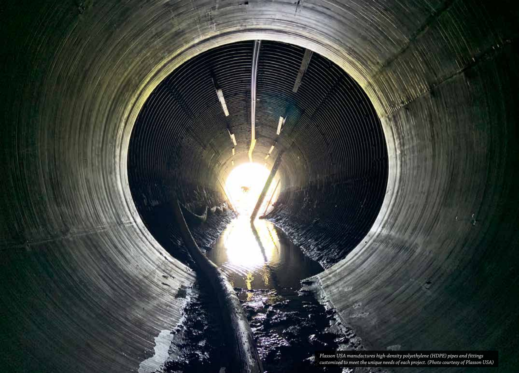
In January 2020, construction workers in Harris County, Texas, installed three 72-inch, 210-foot-long Spirolite culverts featuring tapered ends to fit in better with the natural environment. (Photo courtesy of Plasson USA)
